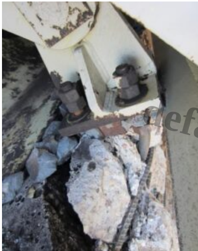
Figure 2: Failed concrete under hinge pedestal.
